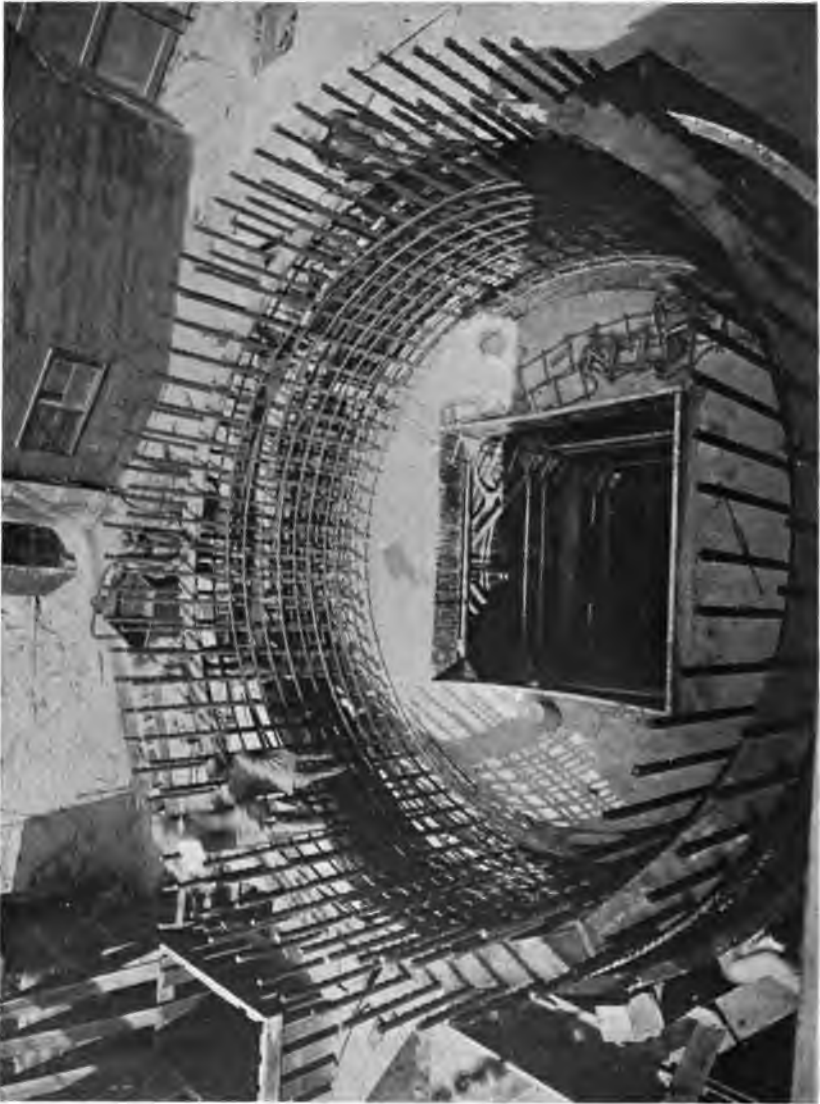
PLATE 227.—Contract 67. View of Reinforcement of Concrete Caissons. Shows also steel outside and inside form and steel platform for placing concrete between forms.
